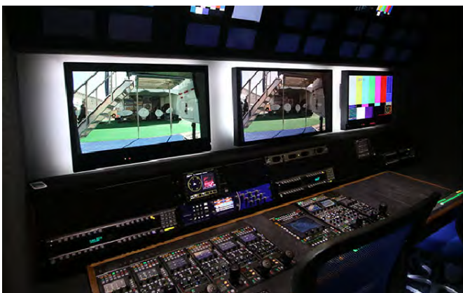
CAMERA CONTROL PANEL
