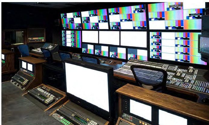
PRODUCTION CONTROL ROOM
