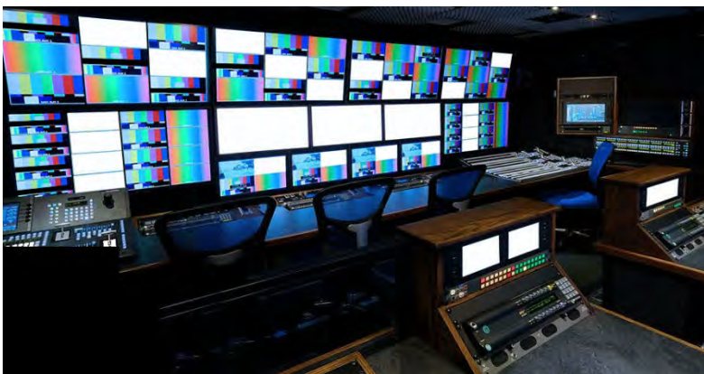
PRODUCTION CONTROL ROOM
